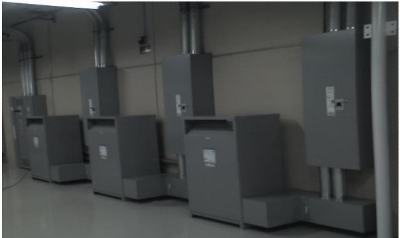
Step Down Transformers 480v to 208v/120v
